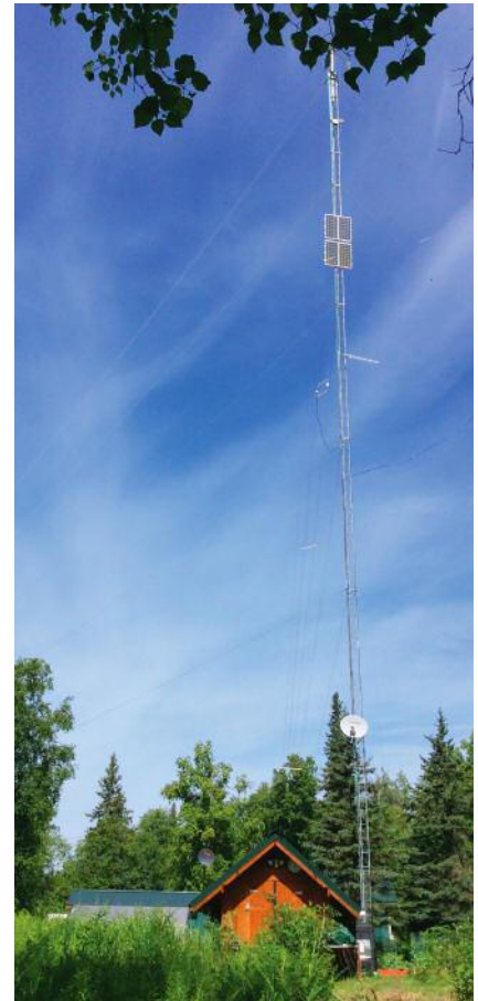
The Emersons installed a 125-foot steel wire communications tower, which both rely on for work and Bryan Emerson uses for Civil Air Patrol purposes.
